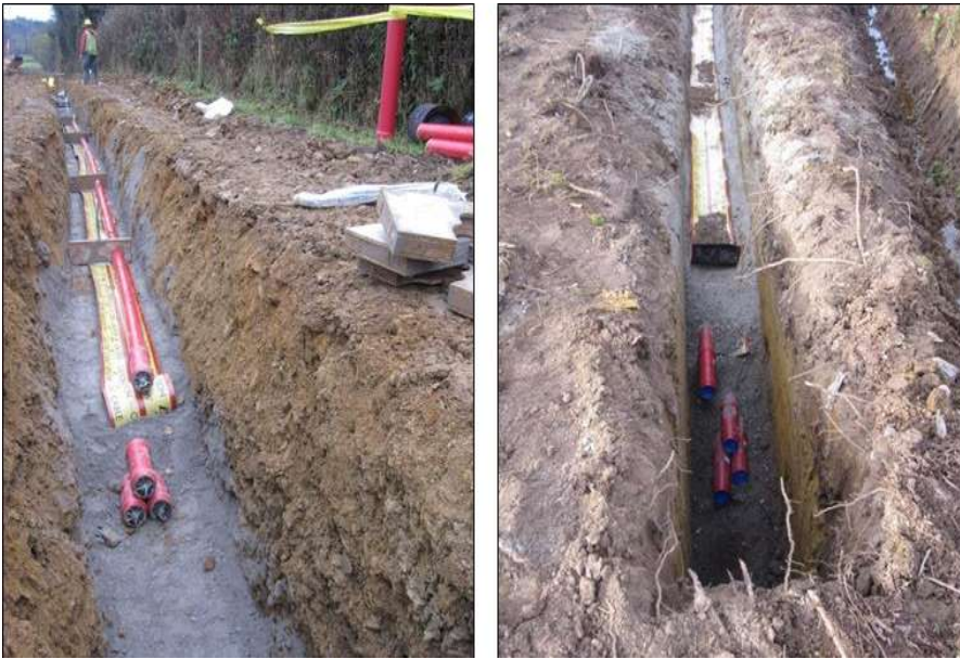
Plate 4-9 Typical Cable Trench View
